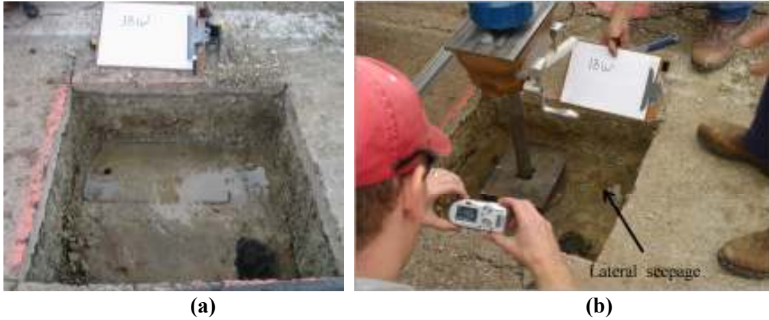
Figure 4.35. Lateral seepage observed in subgrade of Section 13W a) after DCP testing and b) after completion of CBR testing.
