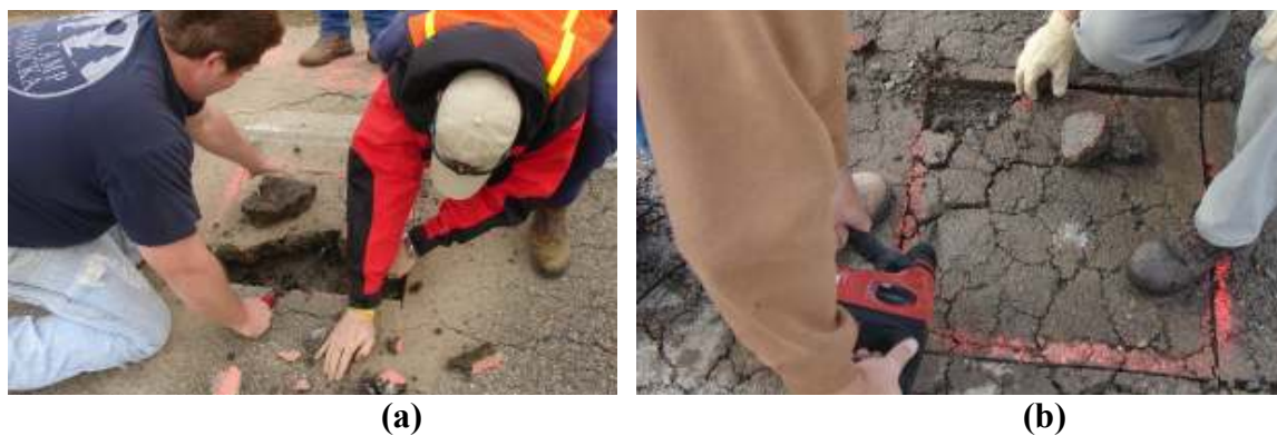
Figure 3.5. Removal of asphalt using a) crowbar (Section 13W) and b) hammer drill (Section 13BW).
