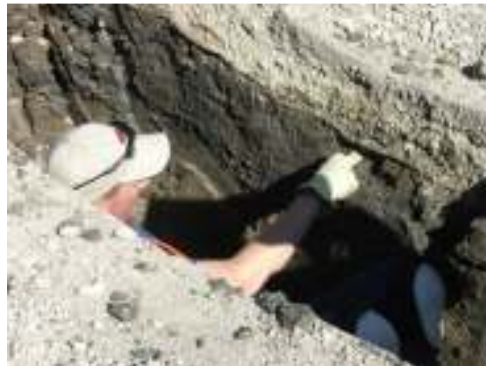
Figure 4.32. Void space observed (Section 13BW) underneath the geotextile.
