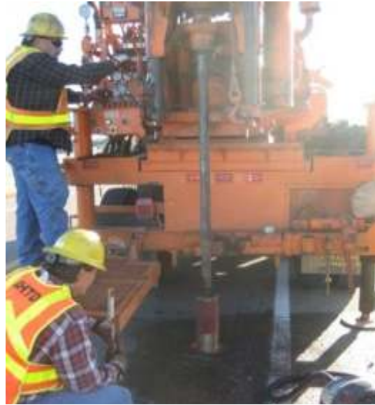
Figure 3.19. Coring by Arkansas State Highway and Transportation Department (AHTD) personnel for installation of two stage borehole test casing.
