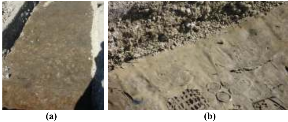
Figure 4.31. Section 13BW subgrade a) after the geotextile removed and b) the zoomed in view after geotextile removal.
